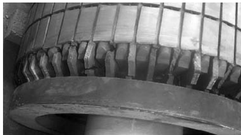
Figure 2.20 Rotor of a 5-MW, 6-kV cage motor with multiple broken bars. © 2017–2018 IEEE. Reprinted, with permission, from Reference [52]
