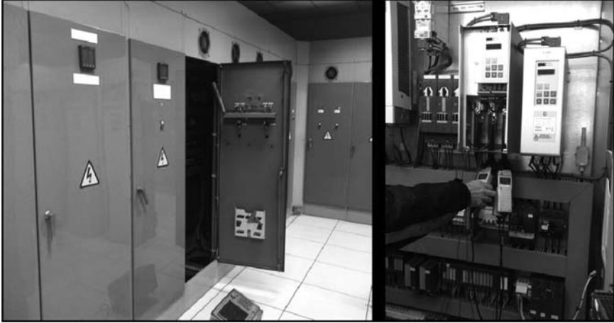
Figure 2.3 Remote monitoring of motor currents. © 2017–2018 IEEE. Reprinted, with permission, from Reference [6]
