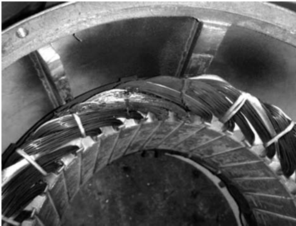
Figure 2.9 Burned out turns of an induction motor's stator winding due to an inter-turn fault (courtesy of Mr M. Thumpy)
